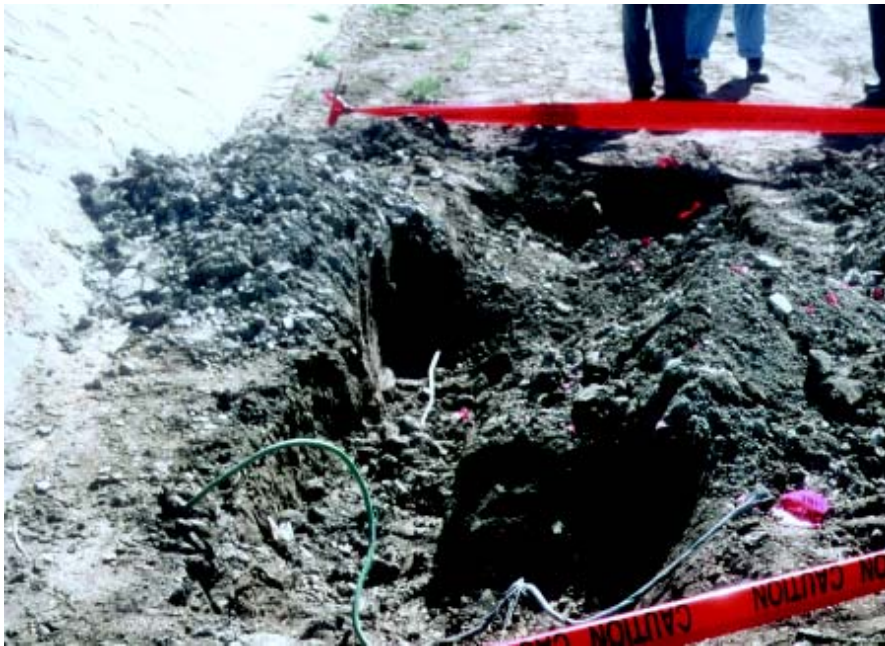
One of many excavations to disconnect bare copper conductors. Green PVC-insulated conductor in foreground is part of the original grid.
