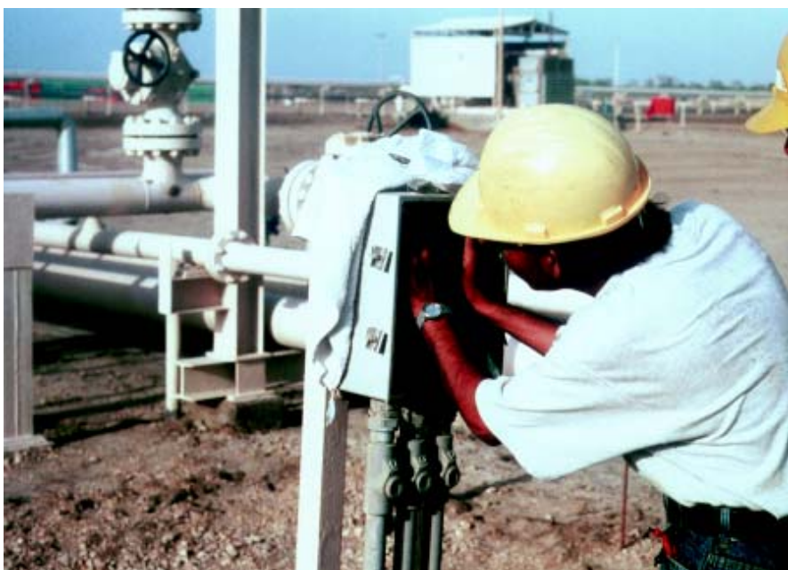
Technician servicing a resistor junction box at the Bukhari Gas Facility.
