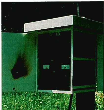
Lightning induced fault current damage to a rectifier door.
